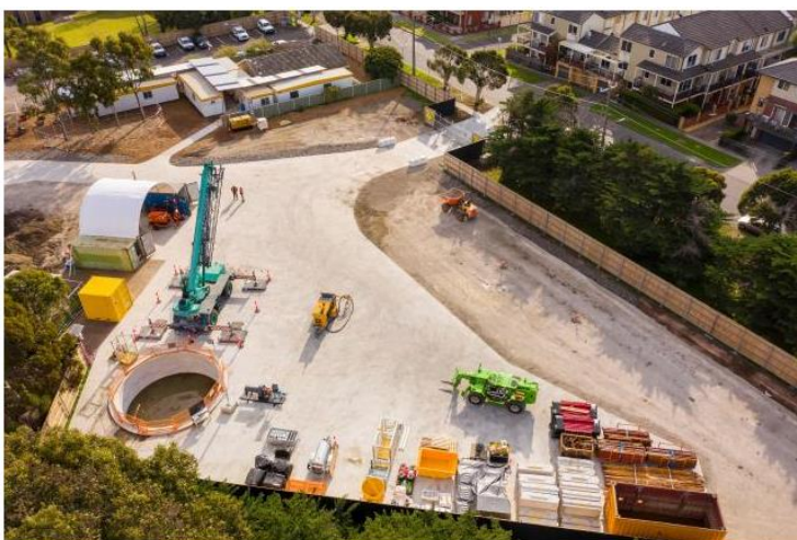
Works are continuing in Maidstone on the Maribyrnong River Main sewer project. (David Hannah)
